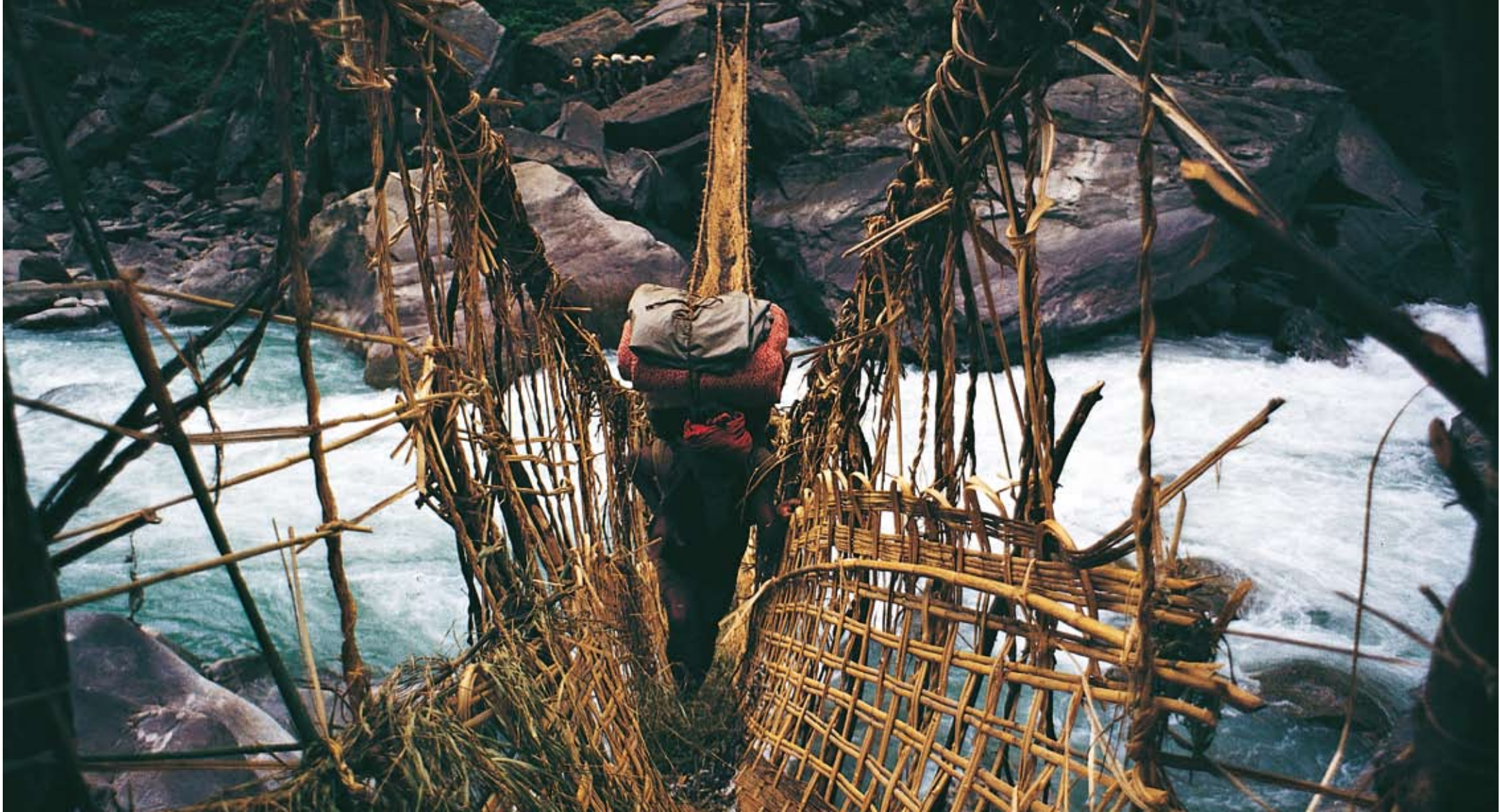
A hanging bridge built entirely of indigenous materials over a glacier-fed Himalayan river. The bamboo matting at the base provides for safety and stability. The holding capacity of the bridge is low as indicated by the porters awaiting their turn on the far side.
